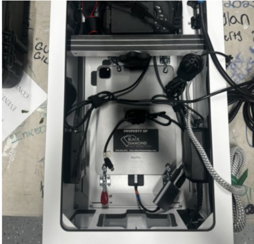
iPad interior — wide view showing cable layout
