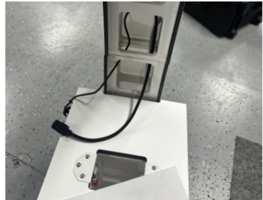
Main power cable exiting at the base plate bottom
